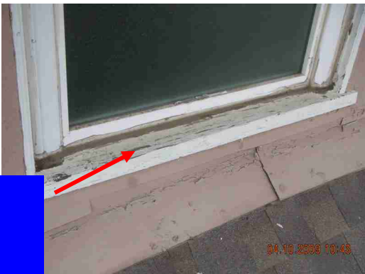
Damaged property wall privacy fence mount
