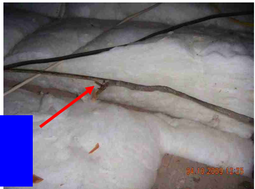
Electrical splice at attic
