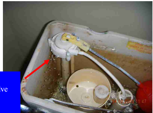
Leak at water heater TPR discharge pipe
