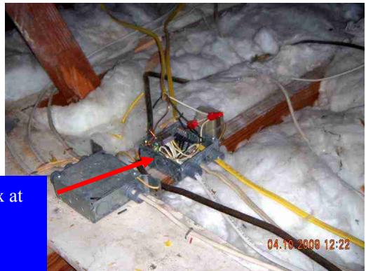
Garage panel has 30 - amp breakers attached to 12-gauge conductors
