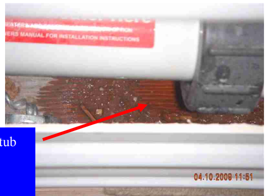
Leak at upper level hall shower cold water faucet
