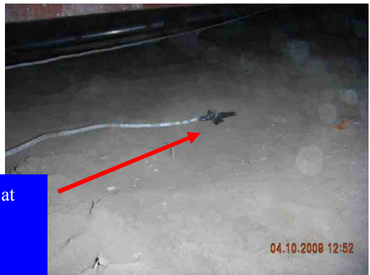
Electrical splice at attic
